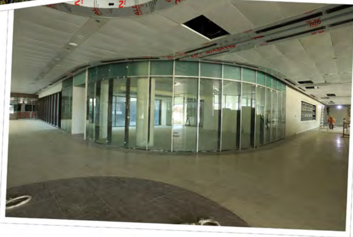
Actual site photos of the new Global Heart Centre, as of December 2024.
